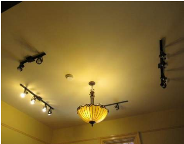
Picture ME 11 Components – Interior CFL lighting Location – Throughout
