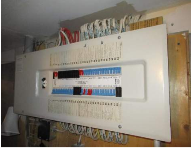
Picture ME 09 Components – Electrical panel Location – Basement
