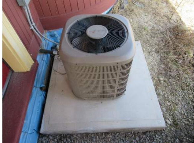
Picture ME 10 Components – Air conditioner condenser Location – North elevation
